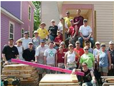
Several Presbyterian Church (U.S.A.) congregations joined together and traveled to New Orleans for home repair. Photo from the collection of Ameer Marks
